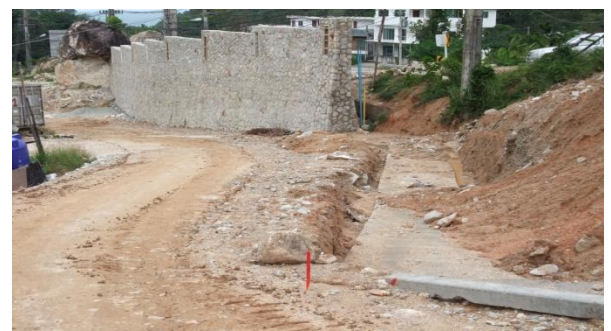
Perimeter wall at lower site area – new guardhouse located to the right of wall foundation
