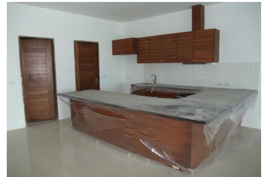
A4-2 Kitchen completed in Makah wood and black granite with bar counter overhang
